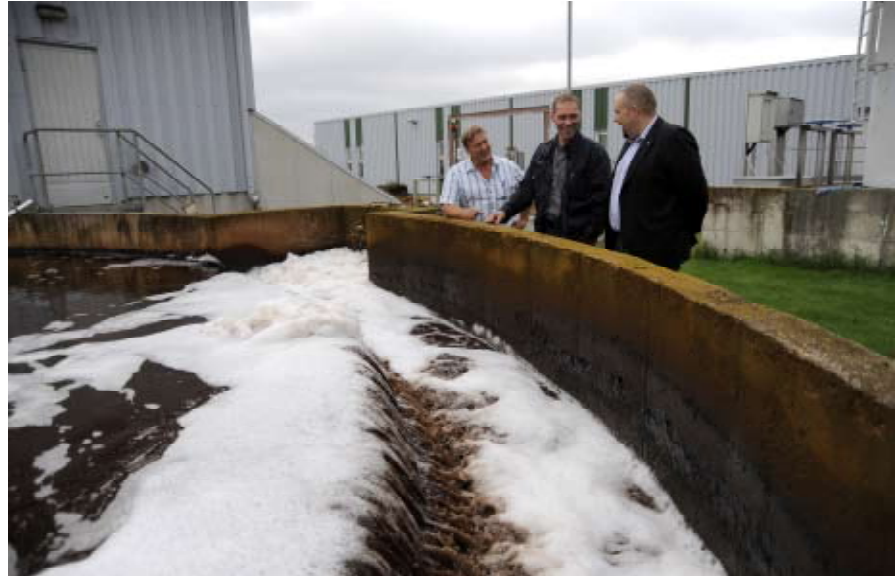
Vesa Hahtokari, plant Manager, Jukka Palomäki, plant Operator, and Jukka Kiiltomäki, Schneider Electric Finland Oy sales Manager, at the activation basin.
